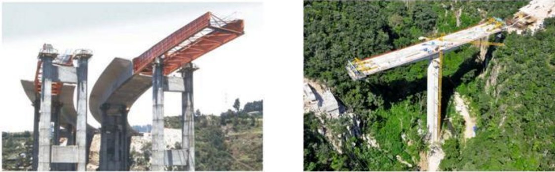
Figure 1. Bridges constructed by the incremental launching method (left) and the balanced cantilever method (right).
