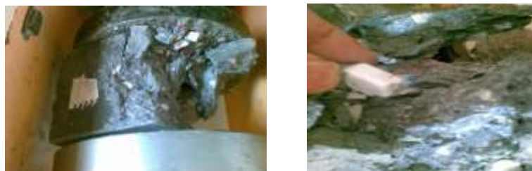
Figure 6, 7. Smooth geometric structure of crystalline calcite inside concrete.
