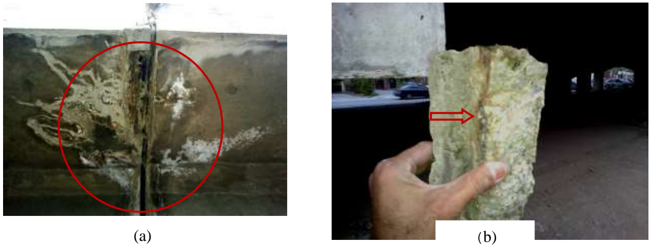
Figure 1.4 Deck Slab of Mian Meer Bridge: a) Unsound concrete; and b) Rust mark
