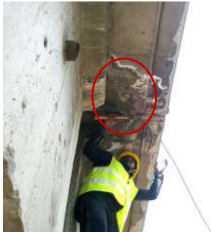
Figure 1.5 Dampness in Deck near Expansion joint in SherPao Bridge
