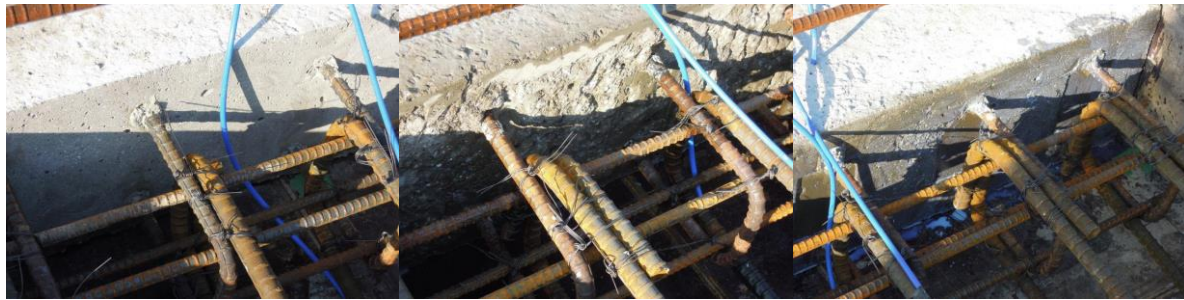
(a) Steel brushing (b) Chipping (c) Coating with bond adhesive Figure 1. Surface condition for interface of specimens
